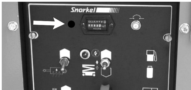
Figure 2.4 - Ground Control Box Alarm
